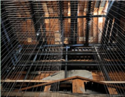
28 lines suspend from our new modern rigging system.
